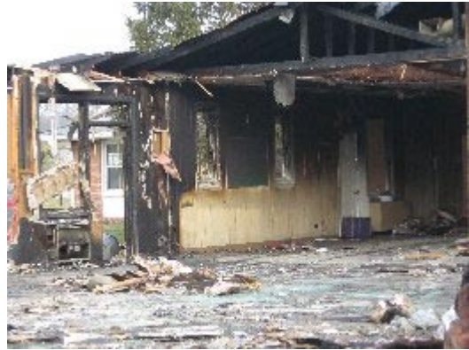
Inside after most of the contents were shoveled away.
