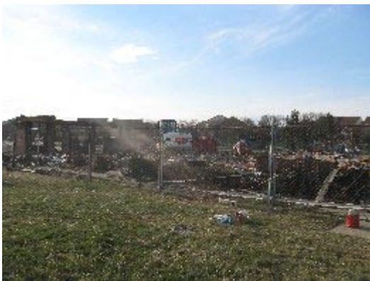
The rubble pile
